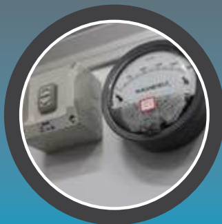
Magnehelic gauges and service lights
